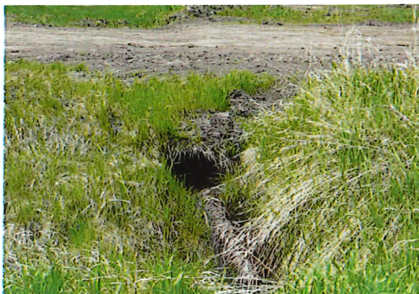
Culvert blocked by grass/debris
