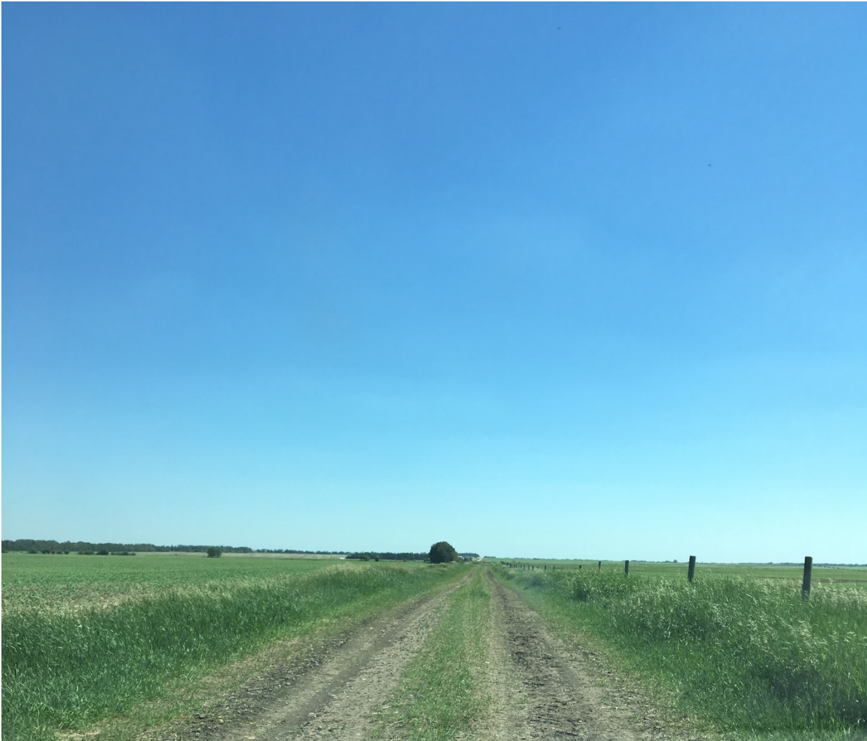
Figure 5-2 - Gravel Road in Poor Condition (2) – Rating 3.0
