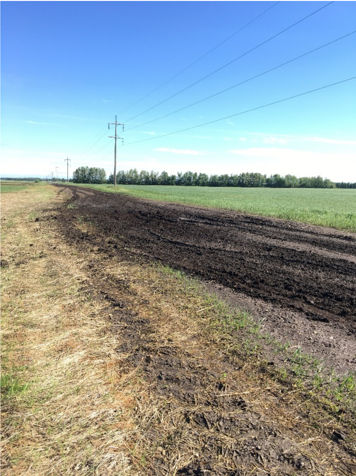
Figure 5-1 - Gravel Road in Poor Condition (1) – Rating 2.3
